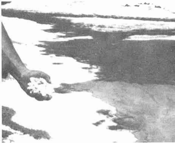
Figure 9. Dolores riverbed. View looking north mid-valley near upstream limit of saline inflow. View is looking at section of river just to the east of the pump test site. C-1244-406-6
