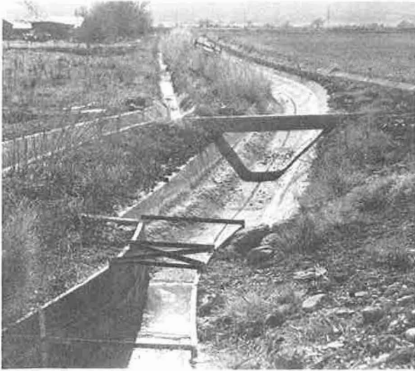
Figure 16. View looking downstream at a small concrete-lined lateral with a Parshall flume in the foreground. The lateral is paralleled by private concrete ditches which are typical of onfarm improvements. P1244-427-45 NA
