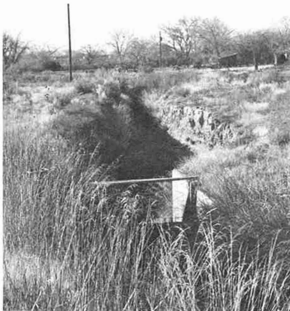
Figure 14. View looking downstream at an unlined lateral from the Government Highline Canal. The measuring device shown in the foreground is typical of the few that are on the laterals. P1244-427-43 NA
